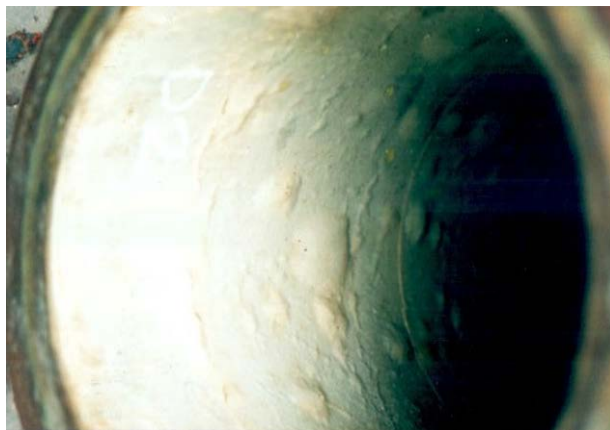
Figure 2.4 Chlorine degradation (left) and HCl induced blistering (right) of a GFRP pipe (Courtesy of AEA Technology)
