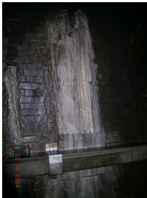
Figure 10. Damp and wet patches, low water ingress
