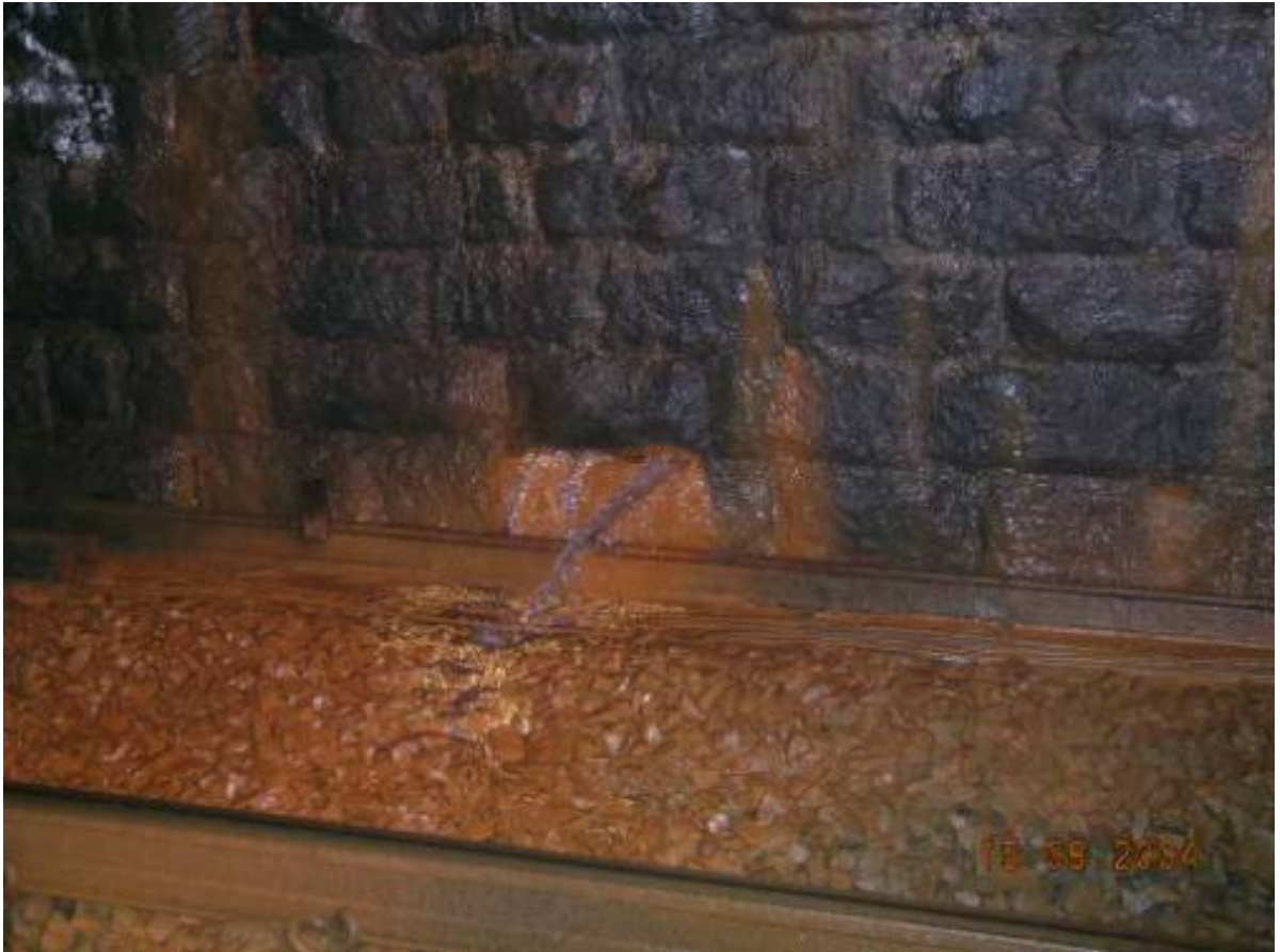
Figure A1.4 Water ingress
