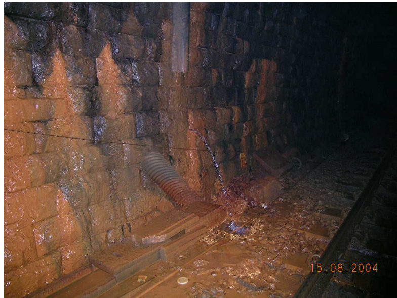
Figure 11. An example of medium water ingress.
