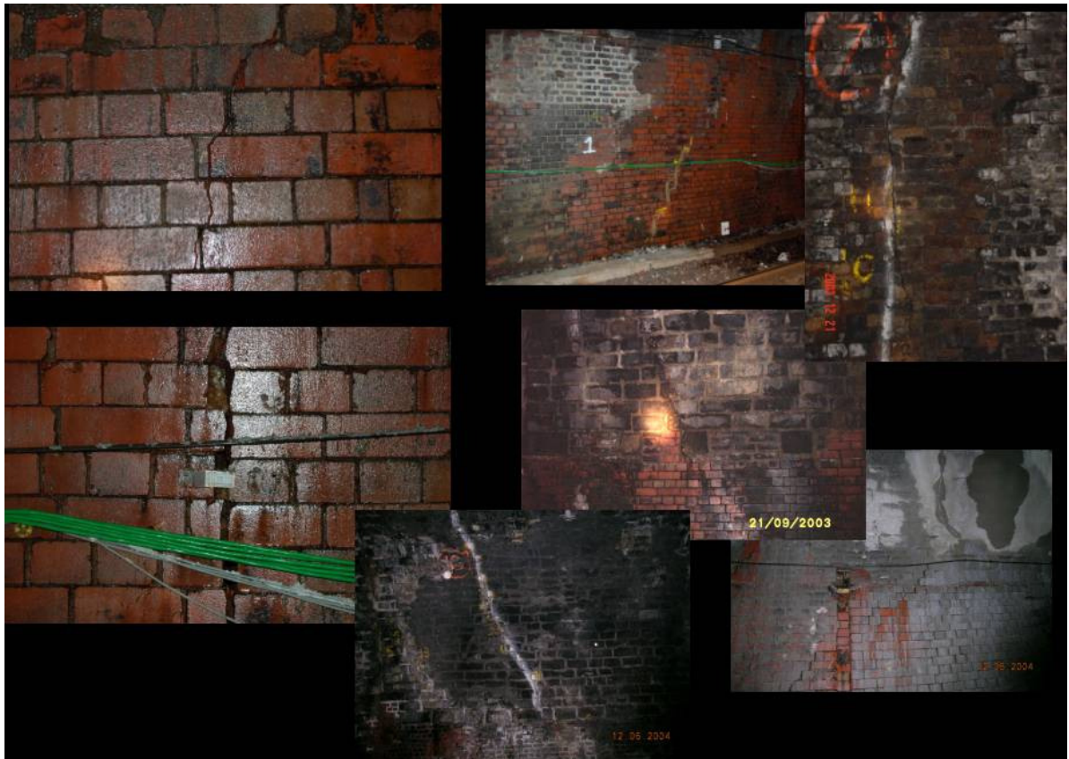
Figure A1.1 Examples of cracking in tunnel surfaces.
