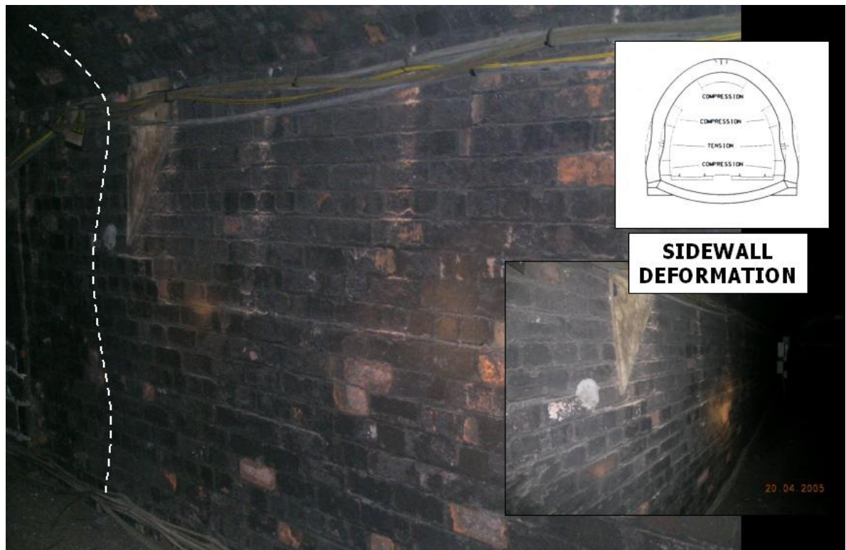
Figure A1.2 Lining deformation (Shape measurement)
