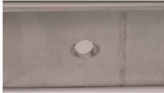
Figure 10: Bolt hole elongation at A.
