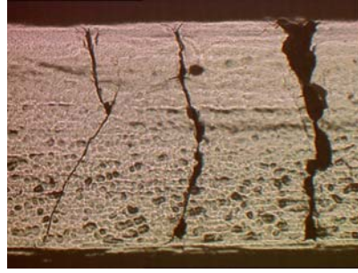
Figure 2: Magnified image of transverse cracks along an edge of a cross-ply laminate.
